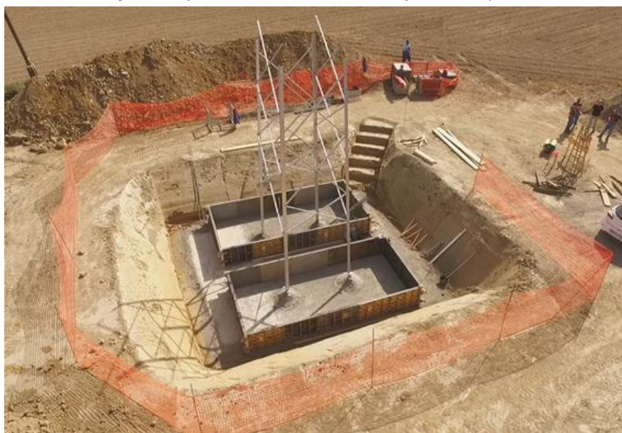
Photo made by drone (Murska Sobota–Mačkovci power line)
