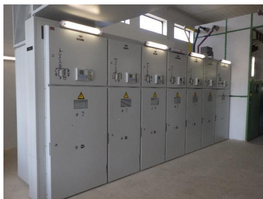
Figure 74: Reconstruction of the DTS Murska Sobota – 20 kV switchyard
