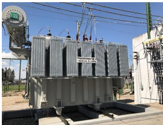
DTS 110/20 kV Ljutomer
