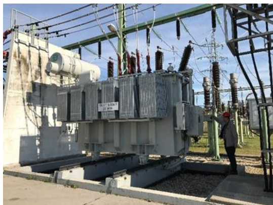
Figure 75: DTS 110/20 kV Ormož
