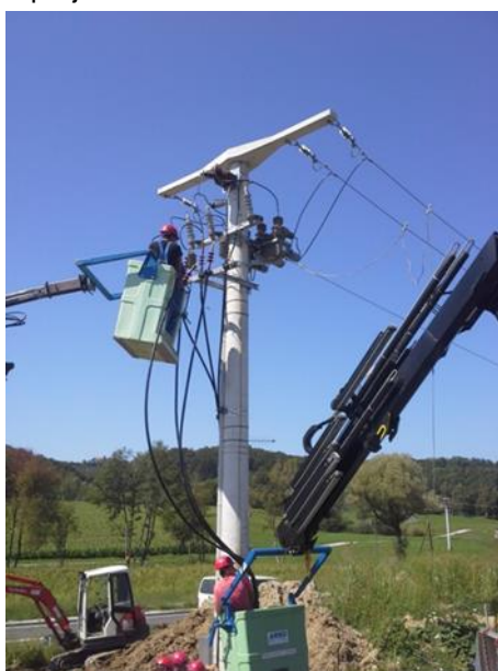
Figure 84: Works of Elektro Maribor d.d. – DMS NEDO project
