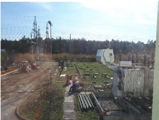
Figure 74: 110 kV RTP Dobrava switchyard
