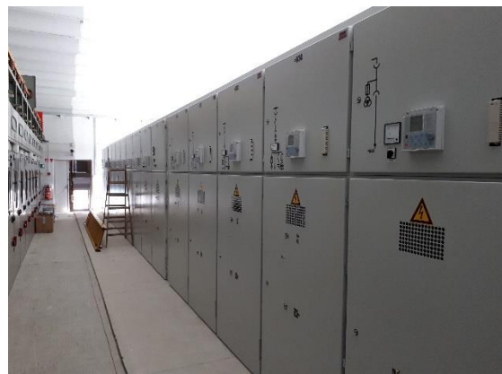
Figure 75: New part of 10 kV cells of RTP Dobrava
