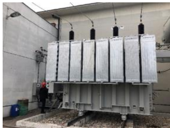
Figure 77: New power transformer in RTP Rače
